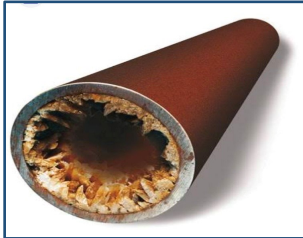
Figure 4. Hard grey scale formation in conveying line.
